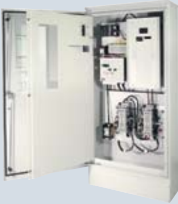
Dual Generator w/ATS
